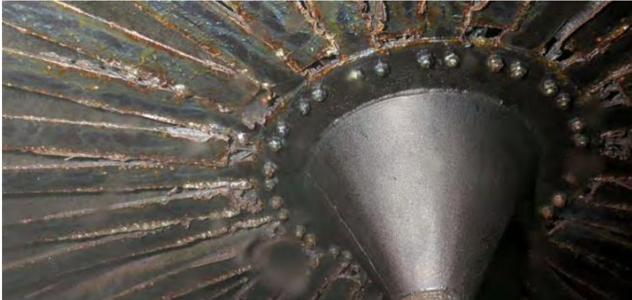
Figure 9-19. Clearwell Interior Corrosion Example (Roof Support)
