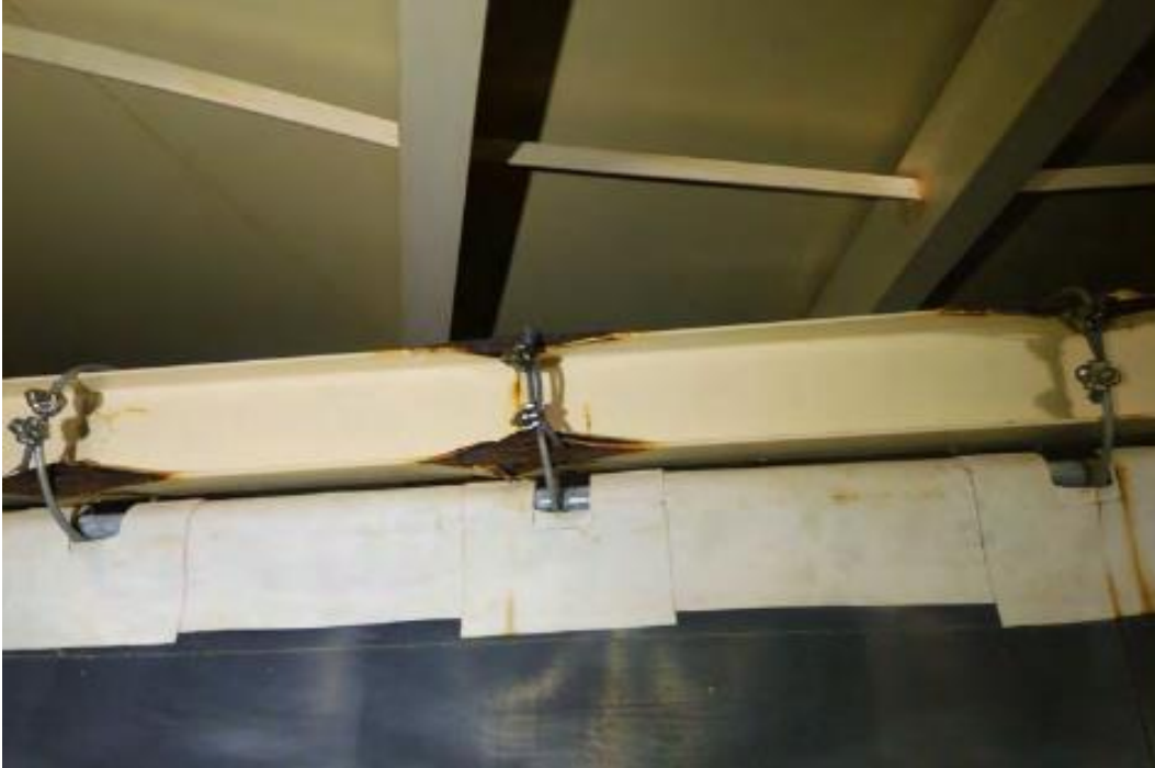
Figure 9-1. Rail Road Flat Tank Dissimilar Metal Location Example
