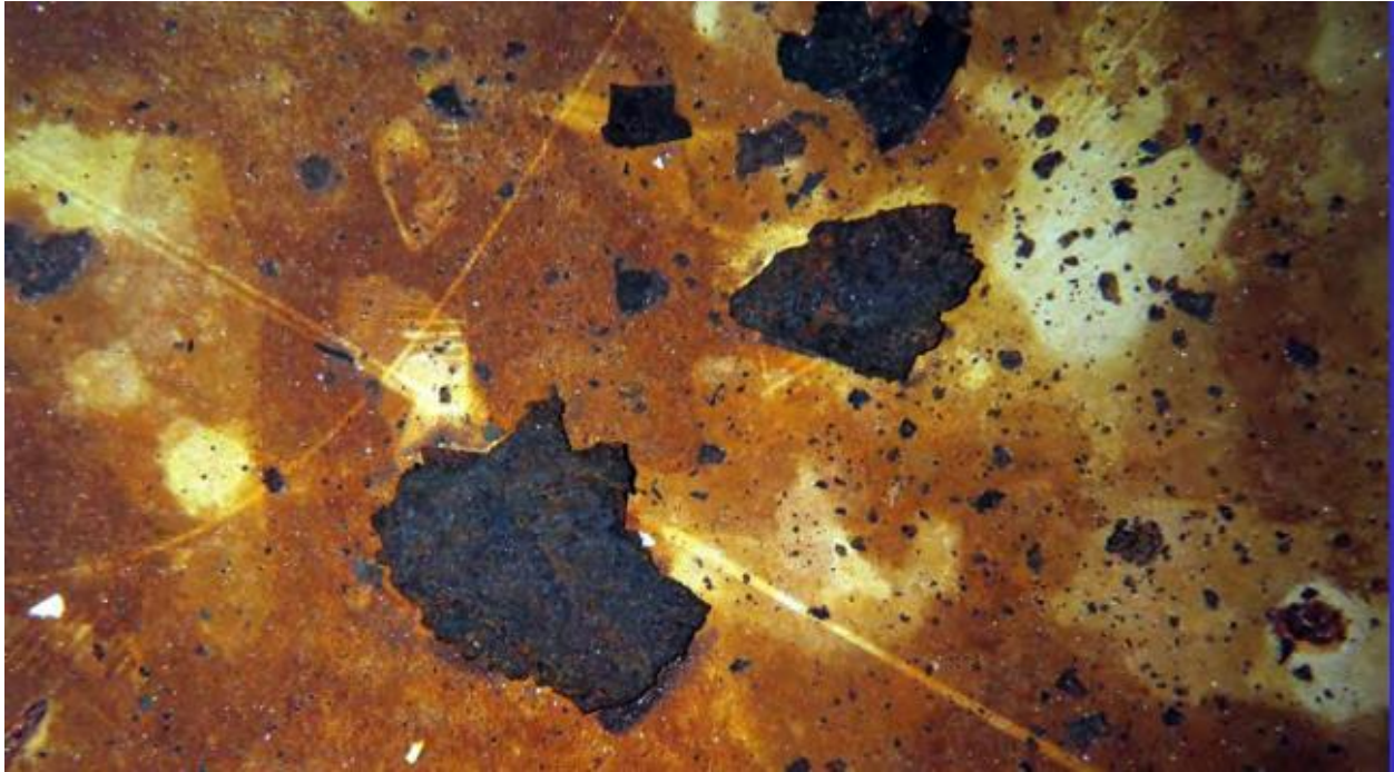
Figure 9-17. Clearwell Interior Corrosion Example (Floor)
