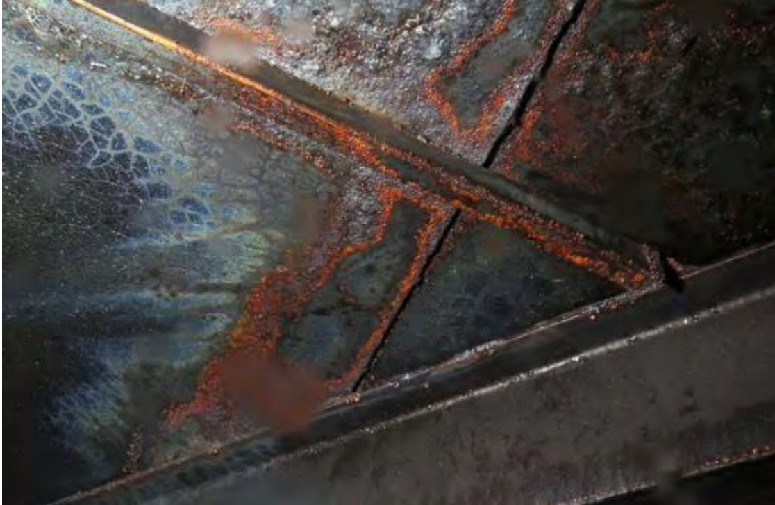
Figure 9-18. Clearwell Interior Corrosion Example (Roof)
