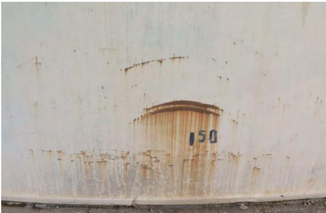
Figure 9-21. Clearwell Exterior Corrosion Example (Sidewall)
