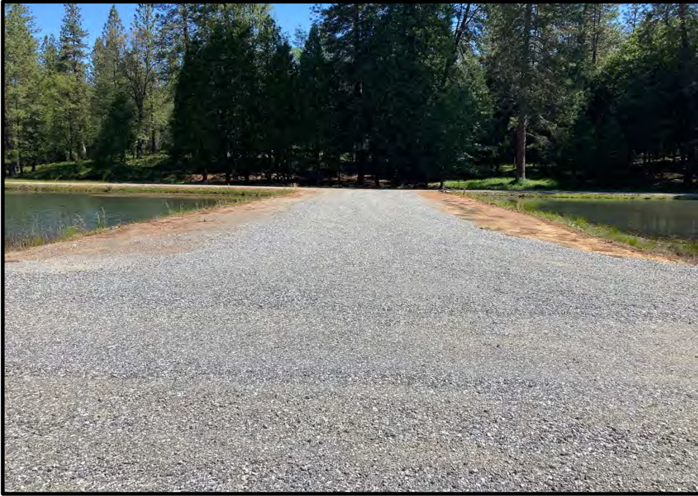
Gravel road between the backwash ponds, looking northeast; 05/15/24. A weir cross drain and electrical conduit serving the backwash recycle pump station will be trenched in this road.
