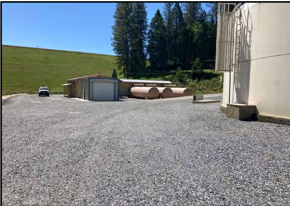
Water treatment plant, looking southeast; 05/15/24. The electrical conduit serving the backwash recycle pump station will be trenched in this road.
